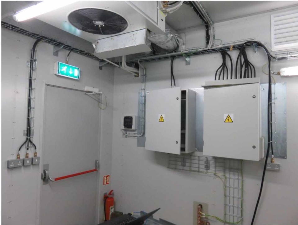
Sample picture which shows emergency light, opening for air-condition, door with panic lock, heating
